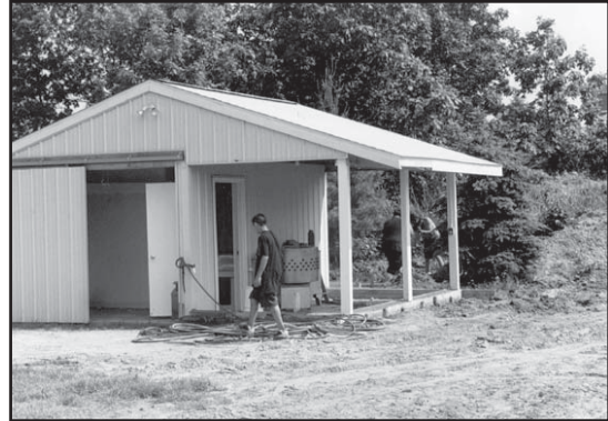
New on-farm processing building on Jones farm (see Farm Profile: Management Alternatives–Day-range).
