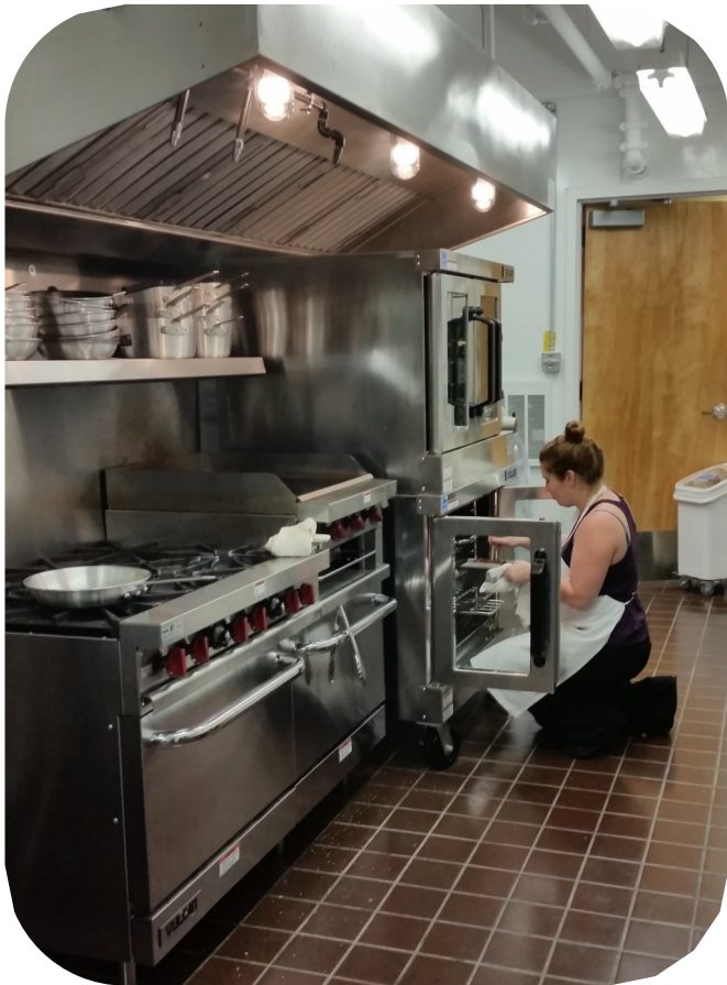
Above: Dining services kitchen at Hampshire College
