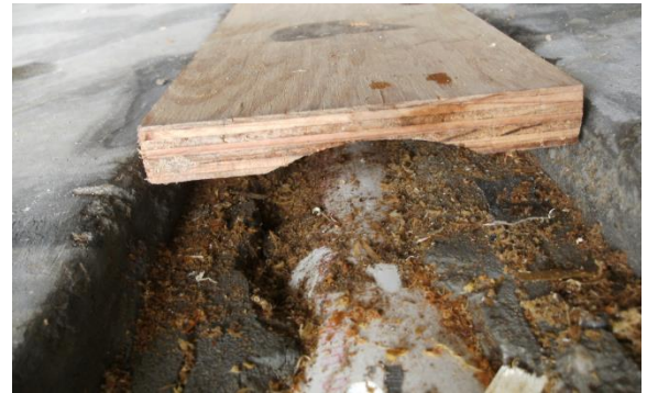
Figure 34: Profile of a Cover Plate over an Aeration Line
