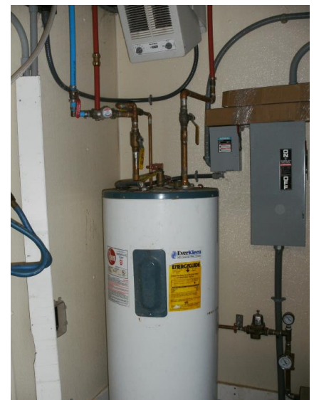
Figure 56: Hot Water Heater Receiving Compost-Heated Water
