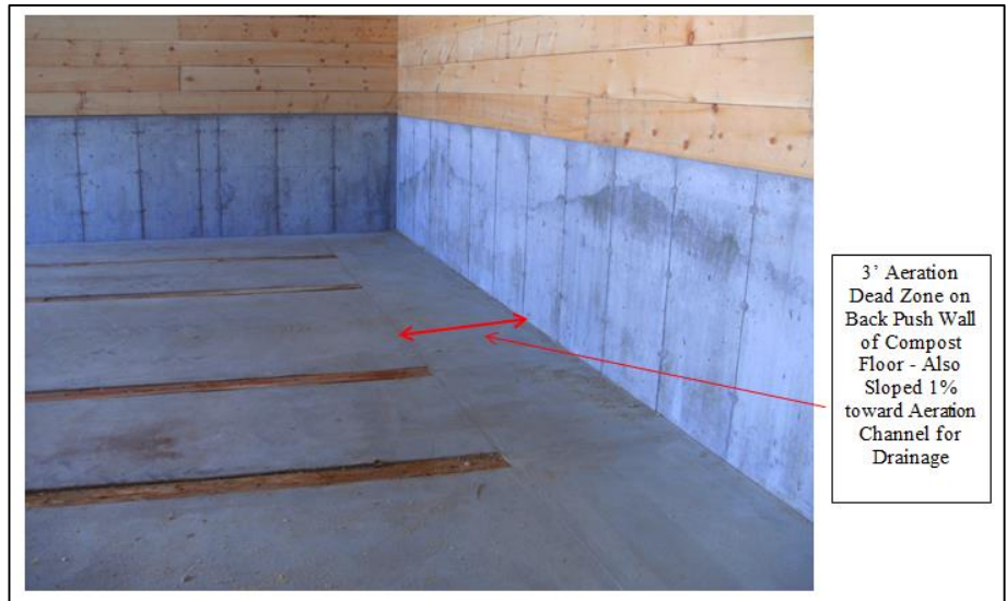
Figure 9: Aeration Line Floor Spacing at the UNH Composting Facility
