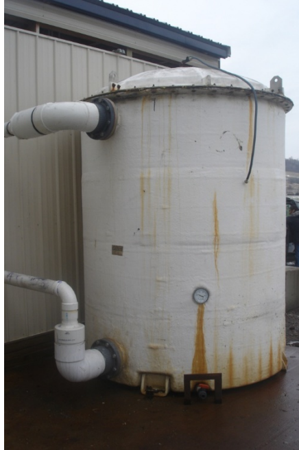
Figure 13. Iron sponge biogas clean-up system on a central NYS dairy farm AD system (Source: C. Gooch)
