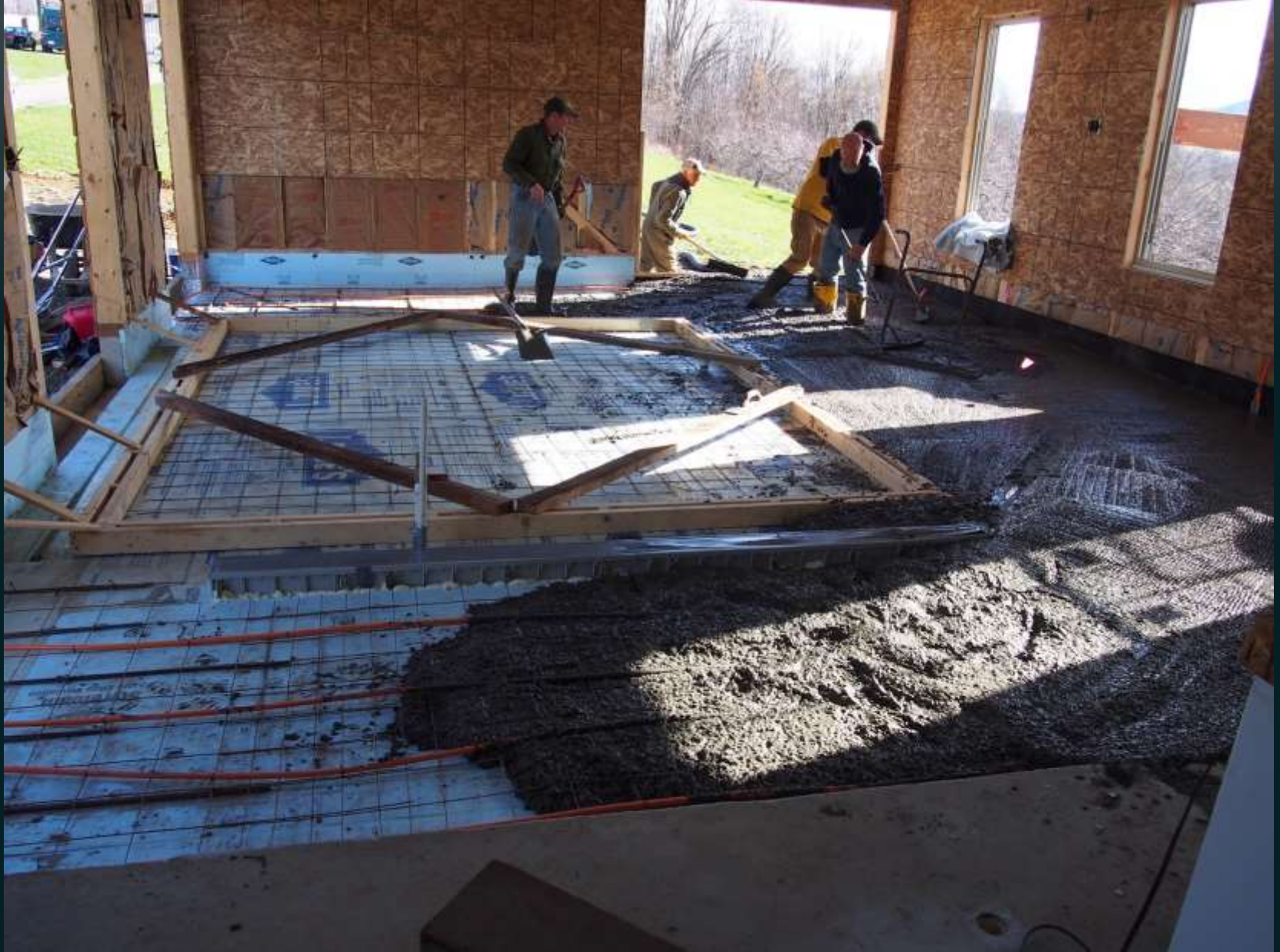
12x14 cooler-Insulation-Radiant Heat
