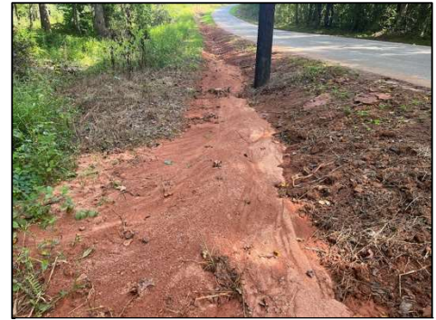
Figure 3. Evidence of soil erosion from relatively small areas of bare soil along roadway ditch. Image credit: Heather Nix, Clemson University.
