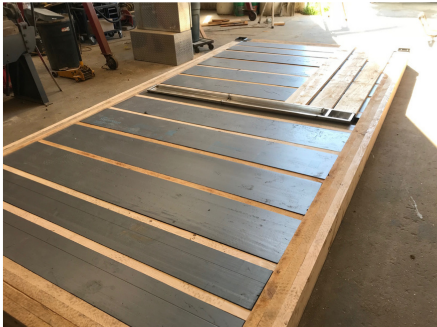
Floor Assembly under construction. Note the XPS insulation in the floor joist cavities. The foam segments sit on nailers added to the joist bases, enabling the foam to provide additional stiffness to the subfloor.
