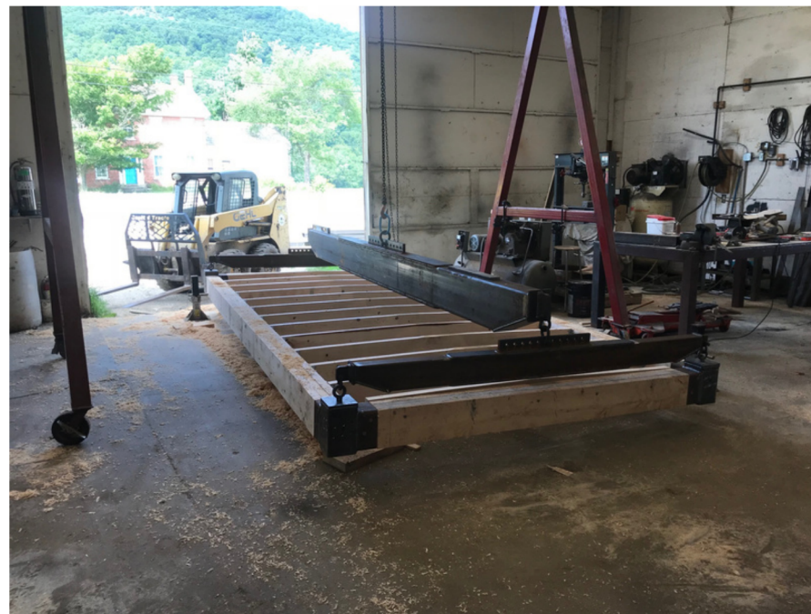
The top portions of a typical ModAPS Core Frame being constructed at The Locust Works. Note the standardized lifting points and dedicated spreader system.
