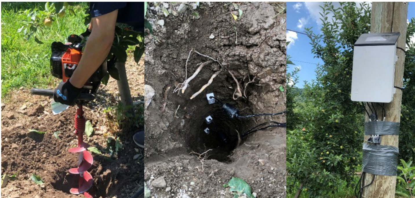
Figure 2. Sensor installation. Dig or drill a three-foot deep hole (left). Install the sensors (middle). Mount the ZL6 datalogger on a post and connect the sensor cables to the datalogger (right). Photos: Long He, Penn State
