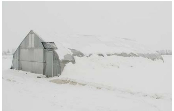
Figure 11. For this structure, snow blocks much of the south sidewall where light would enter, and is also shading the roof. A snow pile on the north side of the structure would provide insulation and not block so much light. (Photo by E. Maynard)
