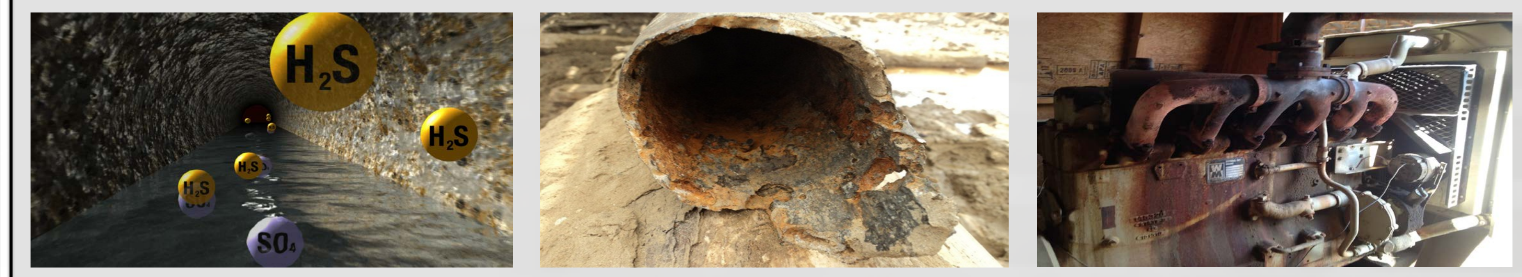
Figure 1. H 2 S production from sulfate rich wastewater (left) and effects of H 2 S induced corrosion in pipelines and generators (middle, right).
