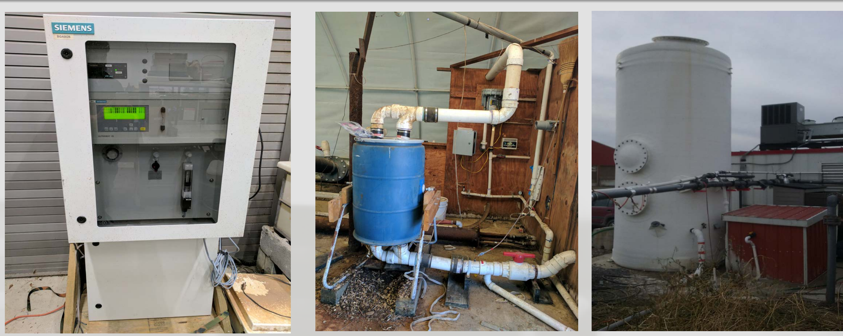
Biogas Analyzer Iron Oxide Scrubber Biological Scrubber
