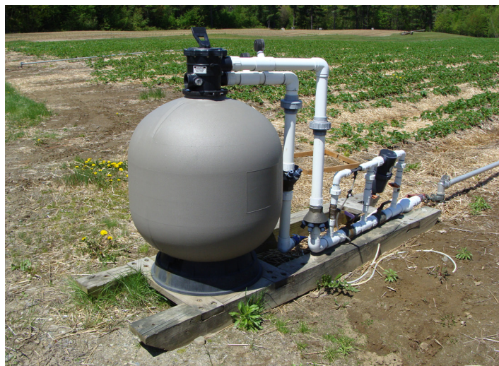
Photo 6-1. Irrigation filter (D. Handley).
