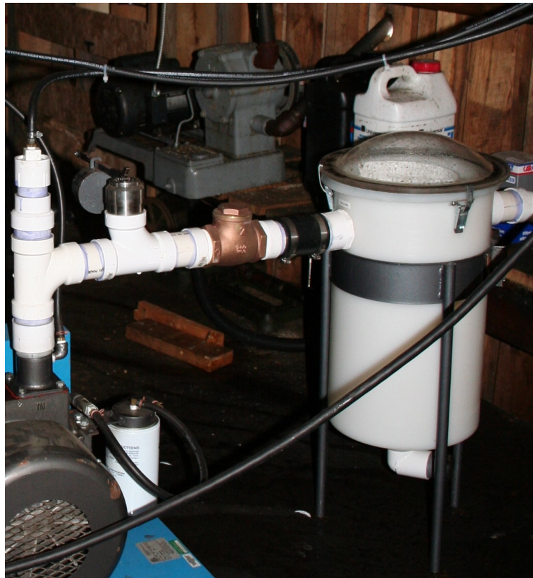
Typical moisture trap, pressure control valve and one way valve
