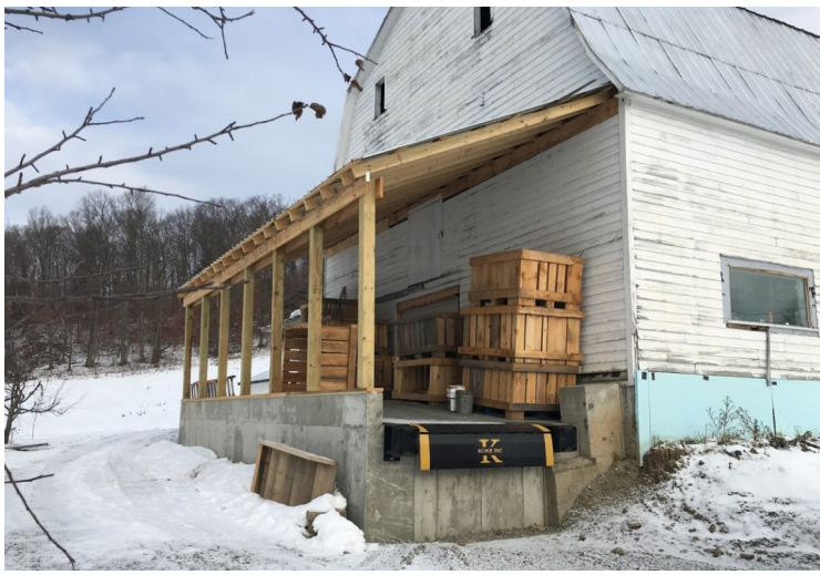
▲ The renovations included installing a covered loading dock, with a dock leveler. This enables easy wholesale transactions and adds additional outdoor covered storage.
