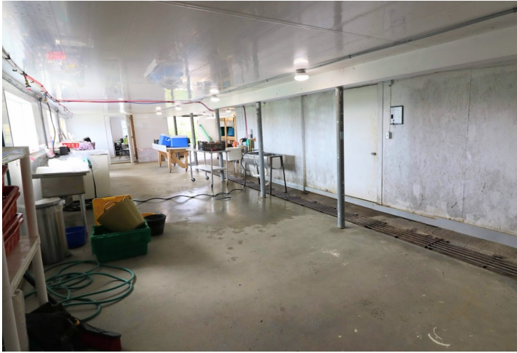
▲ Ceilings are finished with Trusscore , covering up existing flaking paint and enclosing new insulation. Cooler walls painted white, large south facing windows, and an “open” floor plan makes for a bright and useful working environment.
