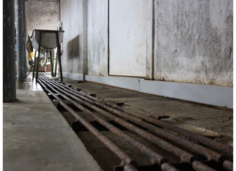
▲ Silas utilized the existing gutter of the dairy barn for wash water catchment. Some chiseling/grading and installation of a clean-out was needed to manage the sediment.
