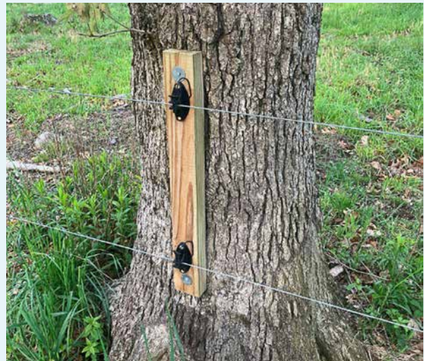
This simple technique can save thousands of dollars on even a small fencing project. Photo courtesy of Ben Coerper.
