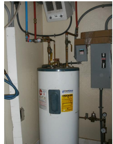
Figure 56: Hot Water Heater Receiving Compost-Heated Water
