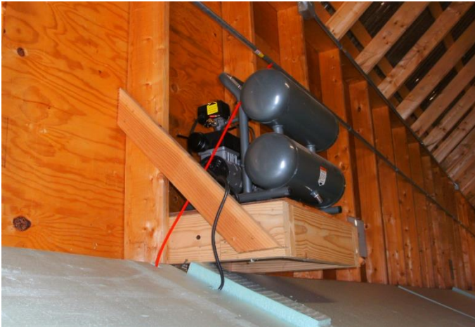
Figure 59: Compressor Running Pneumatic Lines in the Aeration System
