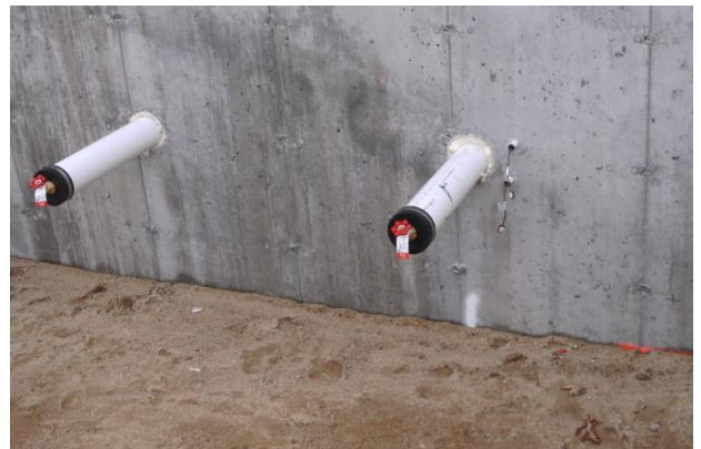
Figure 25: Aeration Lines Through Back Push Wall with Hose Bibbs
