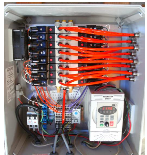
Figure 58: Agrilab's Aeration Control System
