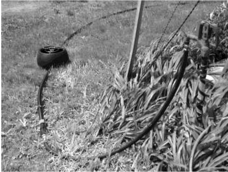
Figure 6: K-Line 1 1/4" tube connected to water hydrant with an AVP 1 air vent in the pod
