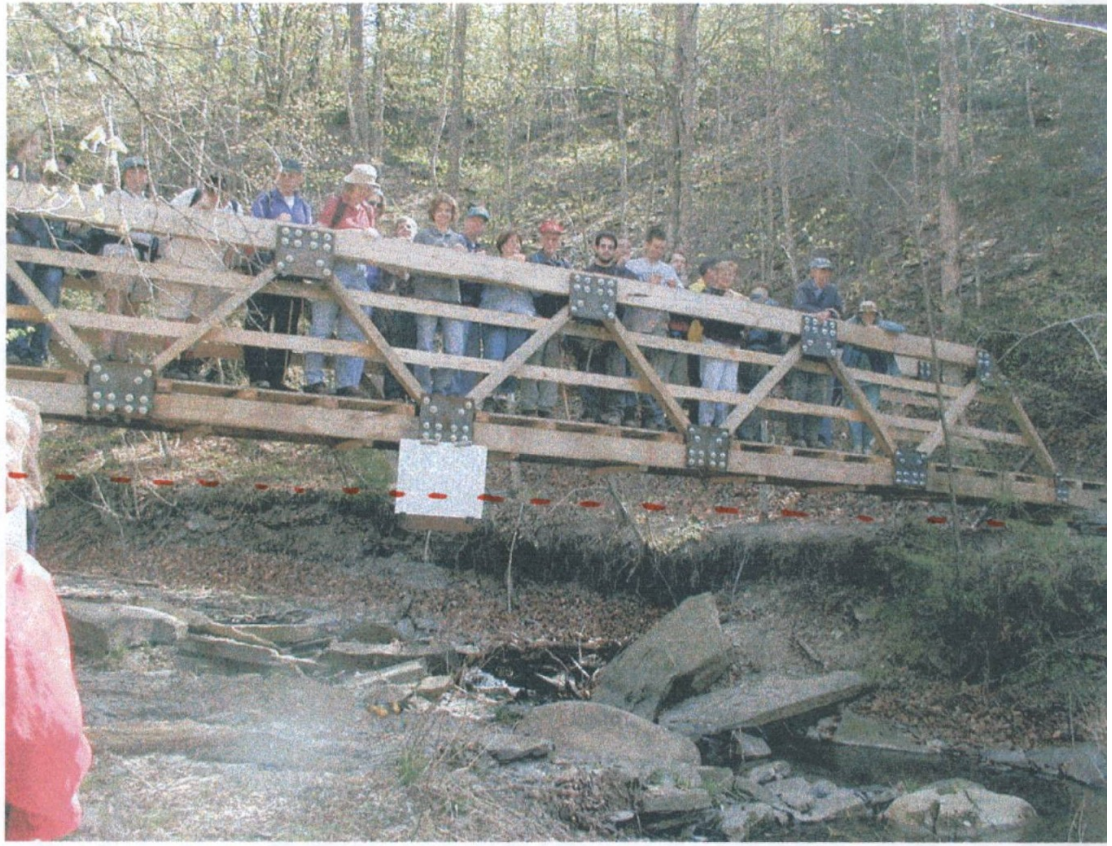
This 53 ft. bridge deflected 1/8 of an inch with 40 people attending the ceremony. A string was tightly stretched from foundation to foundation and at midpoint on the bridge, a white card registered change.
