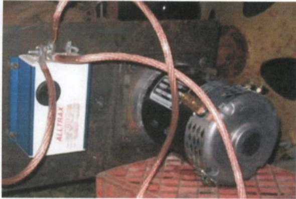
The installed controller. Ignore the wiring for now.
