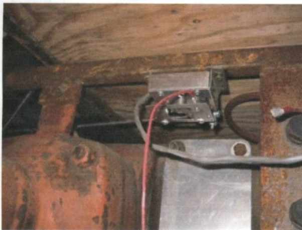
Here is how we screwed the "Potbox" into the metal frame supporting the battery box.
