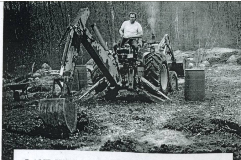
LAND WAS SO ROCKY, I HAD TO USE MY BACKHOE TO DIG HOLES
