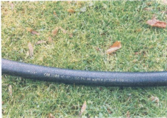
Figure 5. The distribution system leading from the well at the farmstead consists of 1.25" diameter black high density polyethylene pipe laid above ground at the toe of laneway fencing. Thicker walled 160 PSI pipe was actually used.
