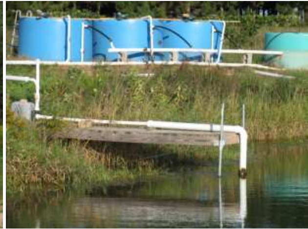
The first three of six tanks. Photos shows inlet, plumbing, and green tank used to collect fish waste and solids.
