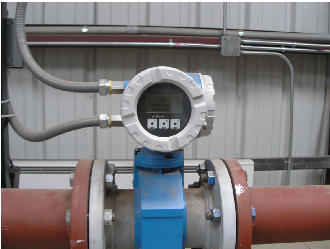
High tech flow rate meter
