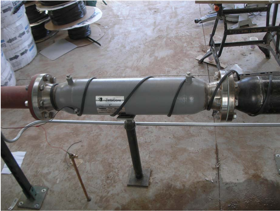
ZetaCore water treatment unit
