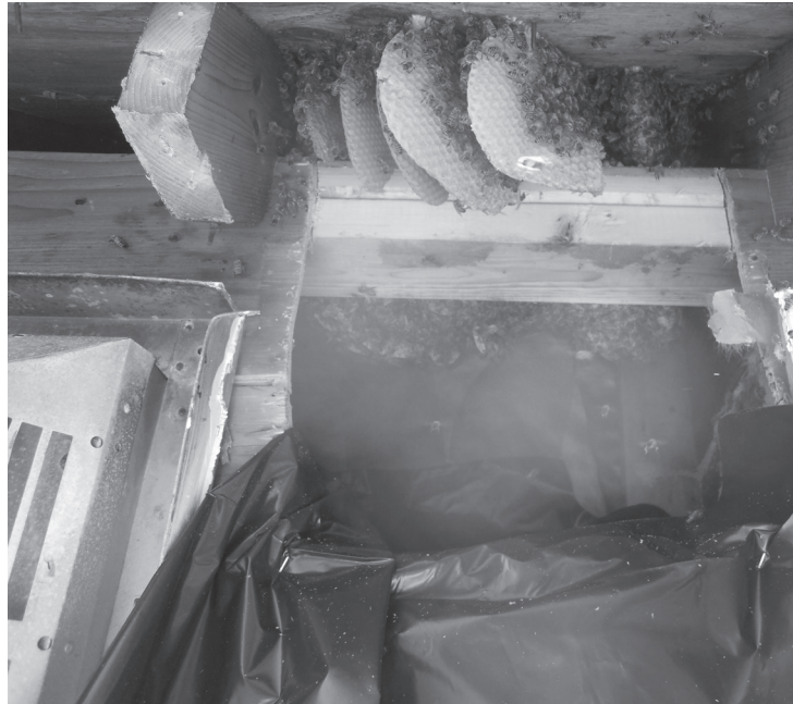
A fireplace bump-out on a Saco home, prepared for the cutout of the colony (approximately 3'x5').
