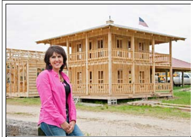
Jo Lynn Mitchell stops near the construction of Tiny Town, an addition to the agritourism venture at Mitchell Farms in Collins, Miss., on April 17, 2014. (Photo by MSU Ag Communications/Kat Lawrence)
