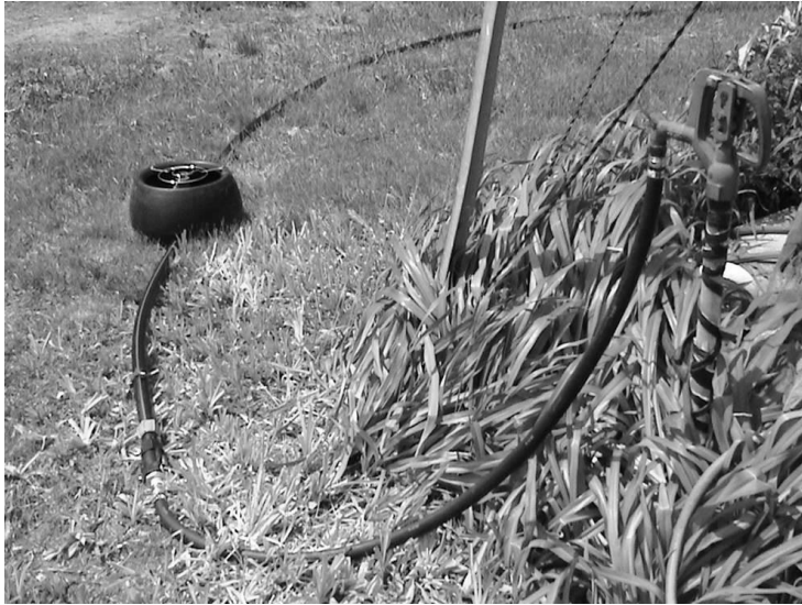
Figure 6: K-Line 1 ¼” tube connected to water hydrant with an AVP 1 air vent in the pod
