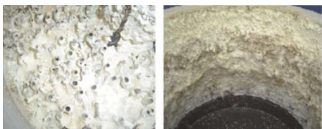
Figure 3: Accumulation of elemental sulfur on the walls and headspace of digester 6 .
