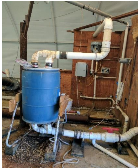
Figure 1. Iron oxide scrubber
