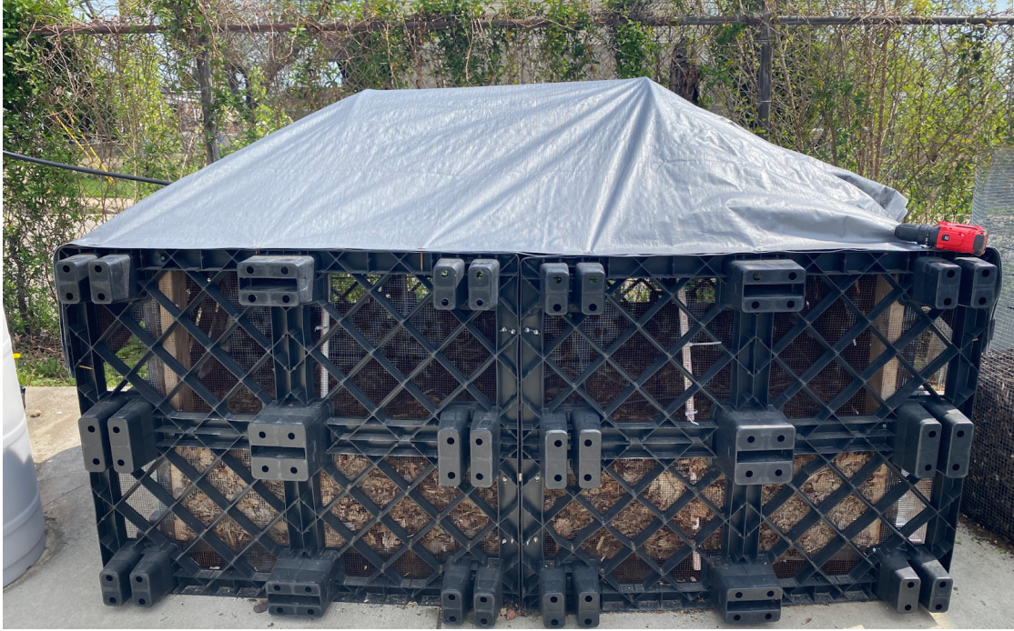
Figure 7. Completed system covered to avoid ponding
