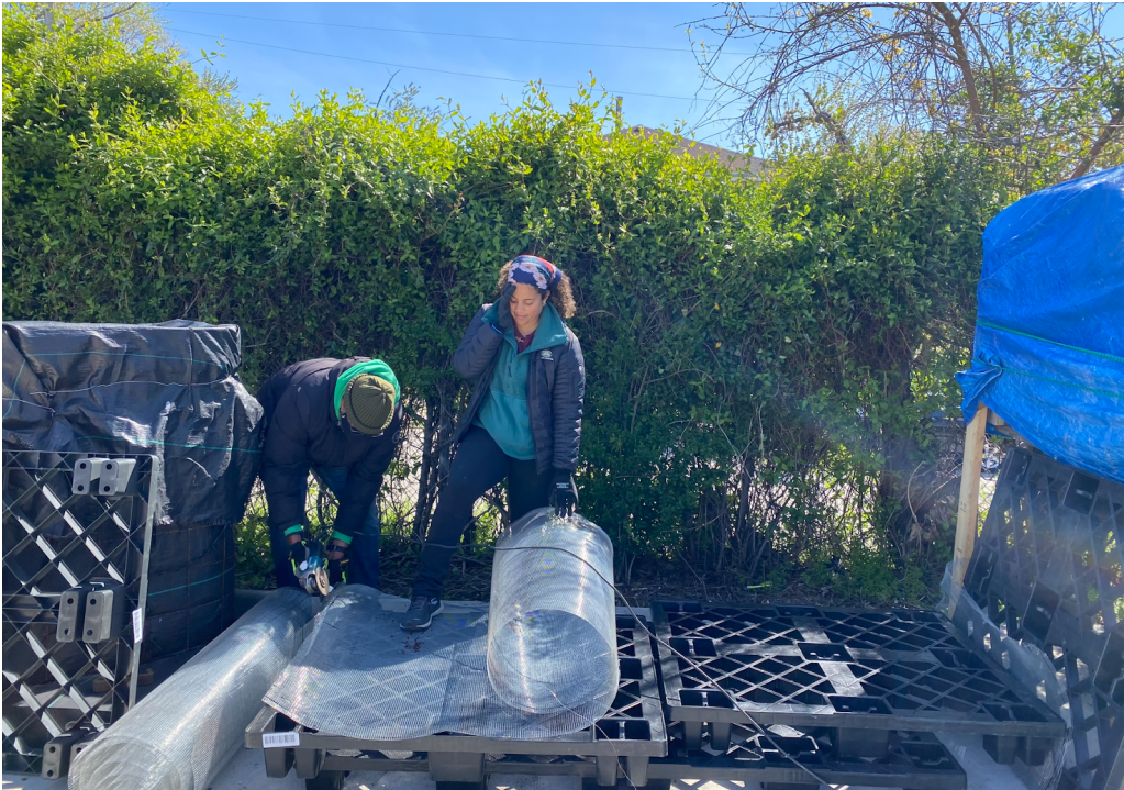
Figure 3. Baltimore Compost Collective and Ridge to Reefs staff building the base for the composting bioreactor system.
