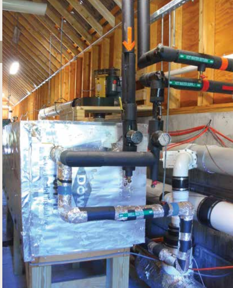
Mechanical room with view of heat exchange unit. Photo courtesy of John Aber
