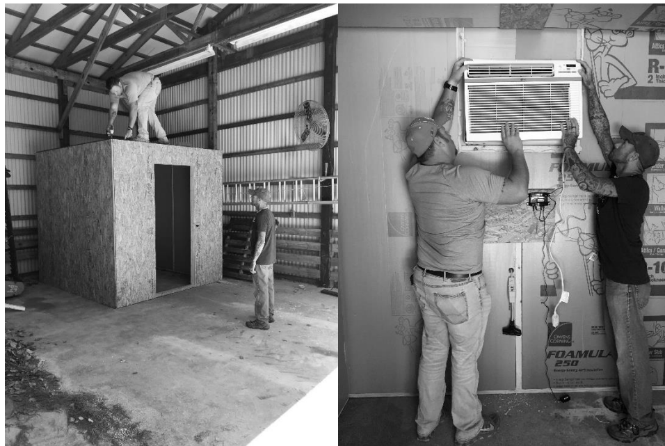
Figure 1. Left: finishing installation of the plywood roof. Right: view inside the cold storage unit while installing the air conditioning unit and CoolBot device.
