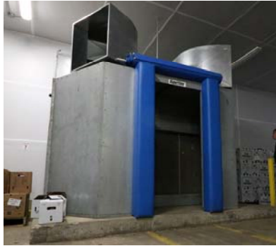
▲ A commercial forced air cooler in a produce distribution facility
